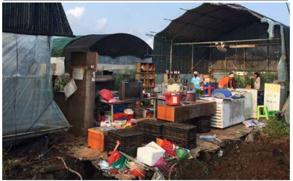
Image by Pang Eunmi. In order to build an access road for the 'civilian' part of the navy base, the Samgeori community kitchen and surrounding buildings were forced out of the way. The kitchen has been cut in half, and the watch tower and houses have been moved.
